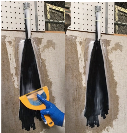
Figure 6 With the insertion tool in place to keep the anchor at full depth, spread the splay end of the anchor onto the substrate. Apply pressure to straighten the fibers with a plastic trowel or similar. Use the syringe to backfill any gaps left by the insertion tool.
