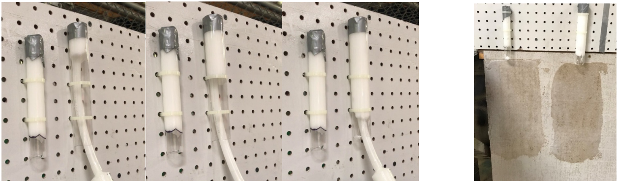
Figure 3 Overhead or horizontal anchor holes are filled with putty with a syringe. Fill from the full depth, backing the syringe out as the hole is filled (left). Prime the surrounding area for the anchor placement (right).
